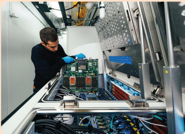
Figure 3 – Full Immersion of servers in a tank
